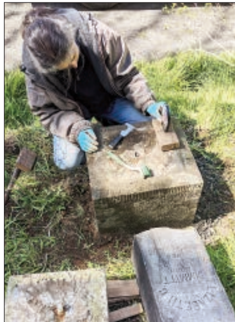
We picked off the epoxy in preparation for lime mortar. — with Bernadette Niederer.
