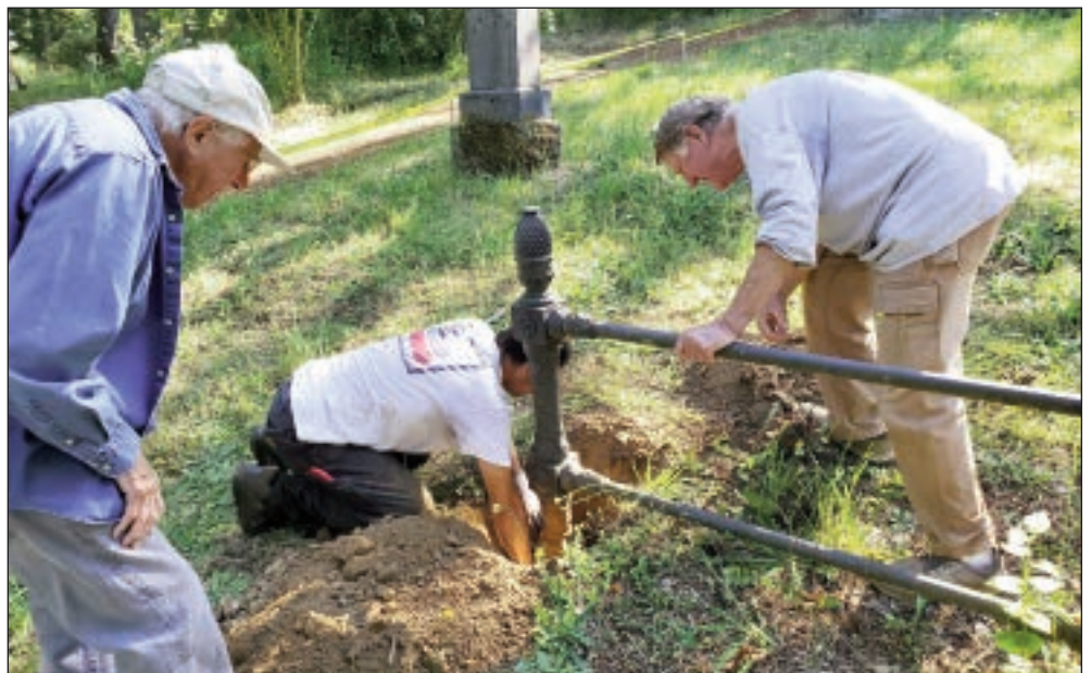
Denny Hellesvig, Diego Llewellyn-Jones and Don Peting working on the McClanahan fence
