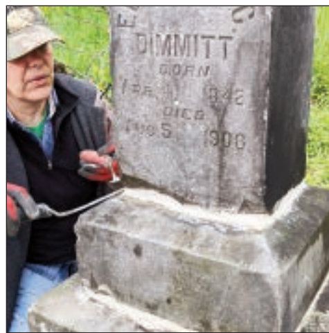
Finishing the mortar. Almost all the stones we work on have lost their arris (i.e., their sharp edges) since they have usually been knocked down once or twice. Therefore, our joints don't come out as sharp lines as we fill the gap to the stone's contours.
