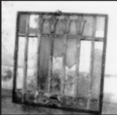
Broken clerestory window
